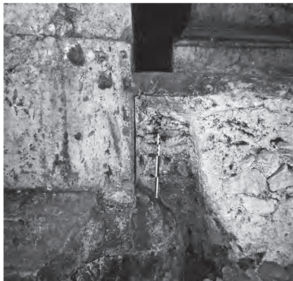
FIG. 6. View from the west, showing how the concrete core of the podium supporting the Augustan base ( upper right ) abuts the southern face of the travertine monument ( left ).
