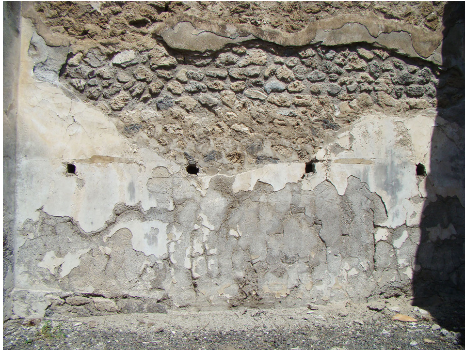
Fig. 8. House VI.13.13, Pompeii, right ala , detail of back wall with holes for shelves (the top row has been concealed by modern restoration).
