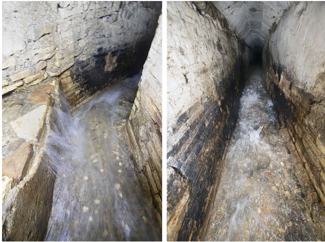
FIG. 7. Views of the offtake channel: left , junction of the zigzag channel (with the higher floor level) and the northern channel, looking north toward the offtake; note the cocciopesto lining of the channel at lower left; right , the offtake, looking northeast (R. Taylor).
