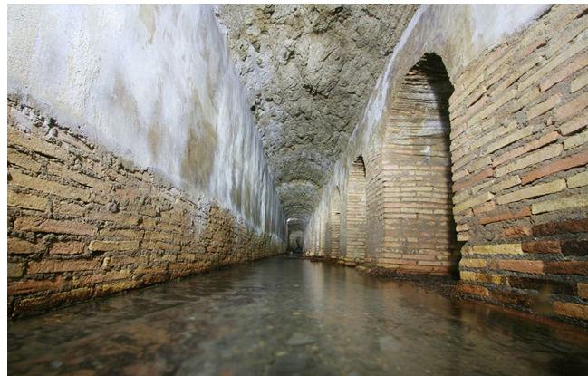
FIG. 3. View of the main gallery, looking south. The wall plaster on the east wall is from the 19th century. Note the absence of plaster from the lower portions of the walls (R. Taylor).
