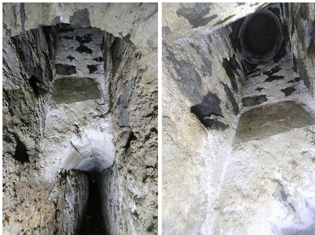
FIG. 16. Pozzo 2, two views from the zigzag channel toward the off-take. Toeholds are sunk into the shaft wall on the left and right sides (R.B. Gorham).
