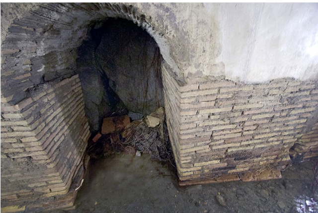
FIG. 6. Arch 13. The bipedales forming the base of Pier 14 (at bottom right) are rotated off the pier's axis (R. Taylor).
