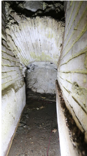
FIG. 15. Ramping vault leading from Grotto 3 toward the middle leg of the zigzag channel, viewed from the grotto (R.B. Gorham).
