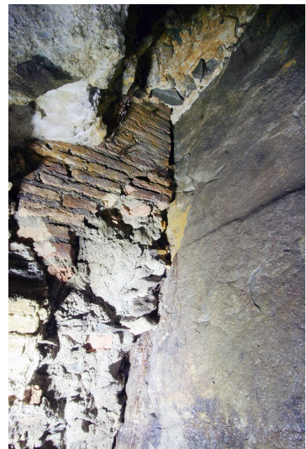
FIG. 9. View into Arch 5, where the ancient brickwork extending Pier 5 to the rock face can be seen (M. O'Neill).
