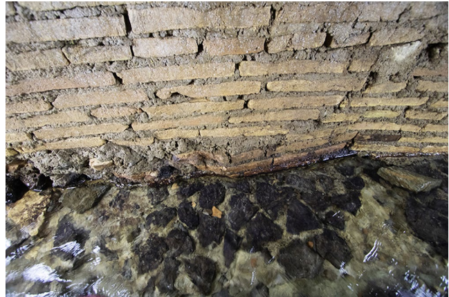
FIG. 11. Detail of brickwork and paving of the northern channel, with evidence of an angle change in the rebuilding of the east wall (R. Taylor).
