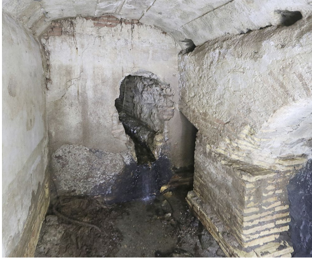
FIG. 1. Junction of the south feeder channel with the main gallery, looking south from the main gallery (R.B. Gorham).
