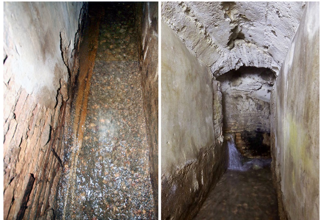
FIG. 13. Views northward along the northern channel: left , the cocciopesto -lined floor as it approaches the offtake; right , the T-junction with the zigzag channel and the offtake (R. Taylor).
