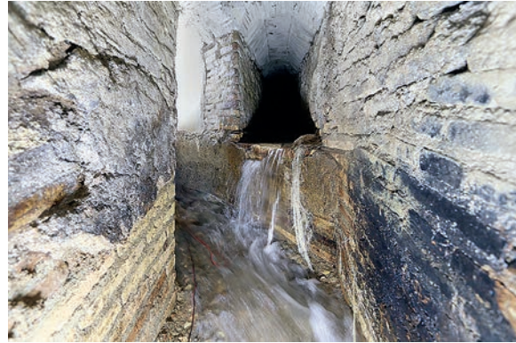
FIG. 17. Junction of the zigzag channel (upper center) and the narrow northern channel (just left of center), looking southwest from the offtake (R.B. Gorham).
