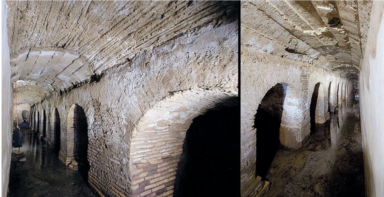
FIG. 16. Two views of the barrel vault of the main gallery: left , the ceiling was bedded on canes; right , on planks (R. Taylor).
